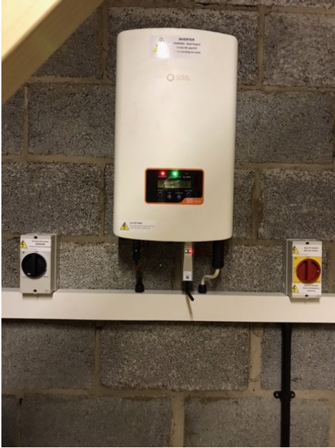
Image 1: The Inverter installed in the Loft
