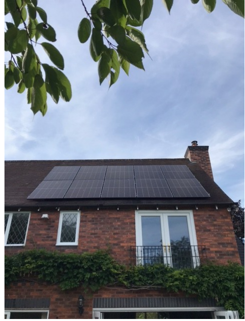
Image 2: Solar Panels fixed to the roof
