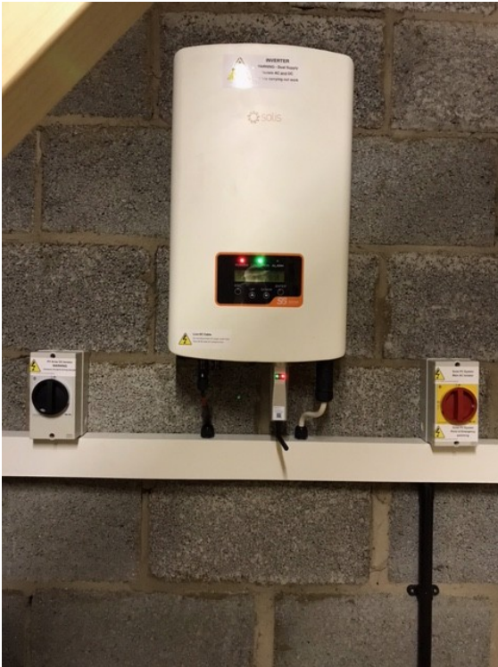
Image 5: Inverter installed in the loft
