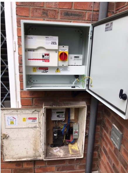
Image 3: The new electrical installation to Support the Solar Installation
